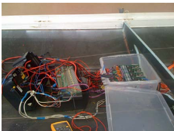
(a) MPPTs in a watertight compartment.
